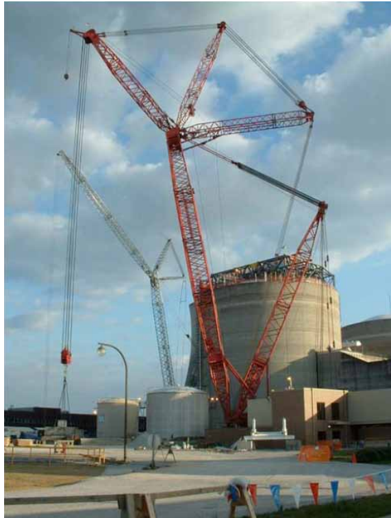
FIG. 23. Outside lift system.
